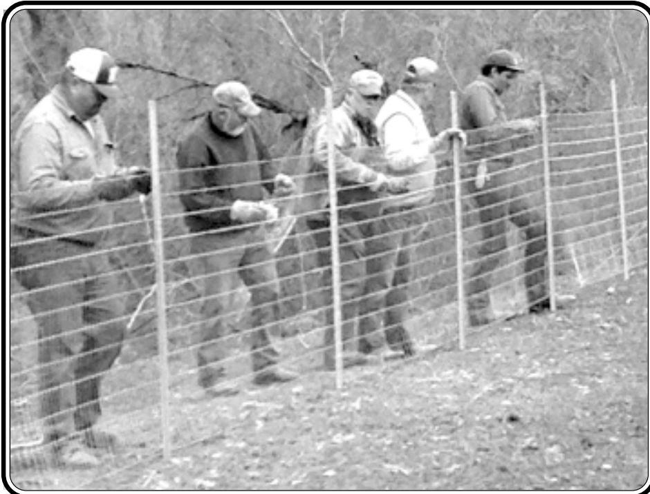
April 16, workers gathered around the new lagoon installing a retaining fence. Pictured are Bill Bickel, Jim Noll, Meryl Lovendahl, Jody Kirkwood
